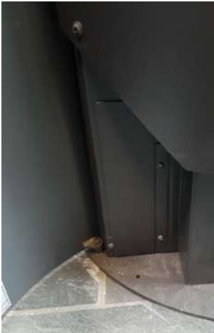
Picture 1: Entry to the control board
